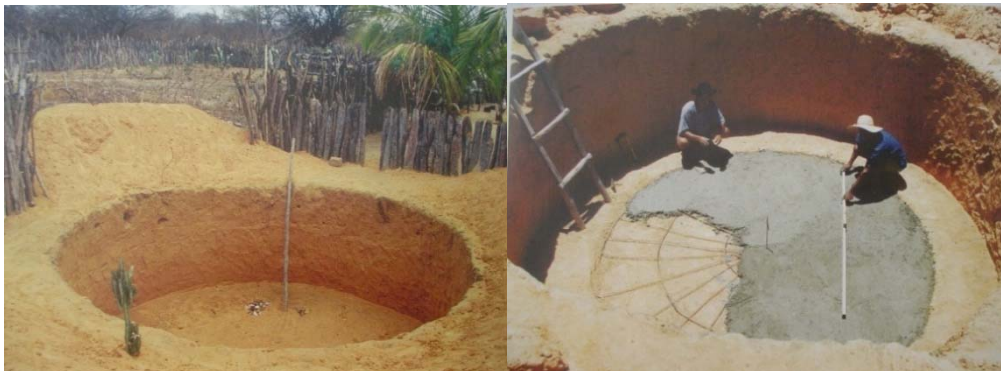
Figure 1 – Excavation of the opening and execution of the concrete flooring of the cistern
