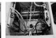
Internal amps and wiring
